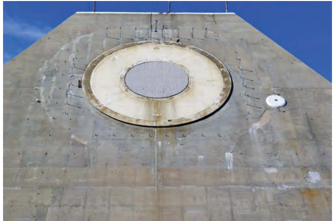
One of the MSCB turret faces showing the radar antenna. The pipes protruding from the face are for the antenna washdown system used to clean or de-ice the antenna. The small antenna to the lower right is the 'Q' antenna which is used to blank the main antenna side-lobes
